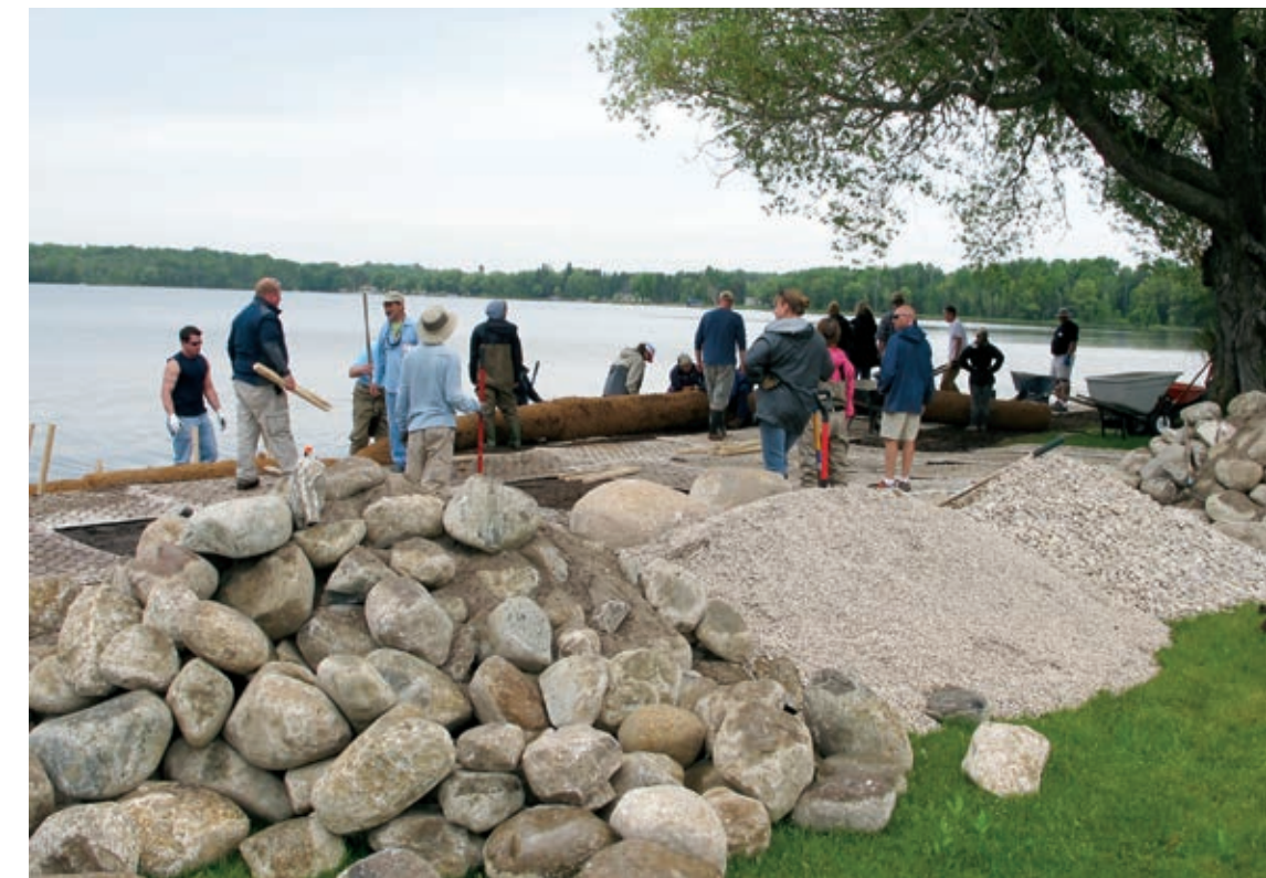
Fieldstone, drain stone, and pea gravel staged prior to installation on a high energy lake. Photo: J. Buchanan
