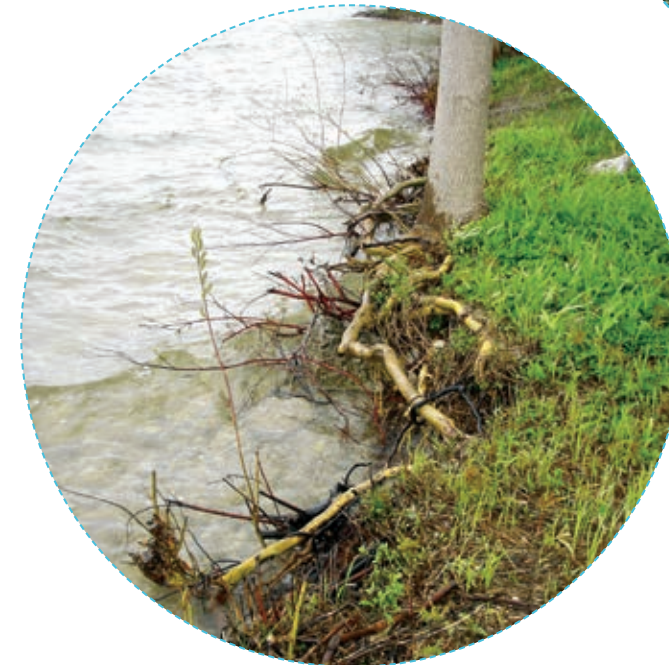
Root Exposure: It is natural to have some roots exposed along shorelines, however, pronounced root exposure is a sign of accelerated erosion.
